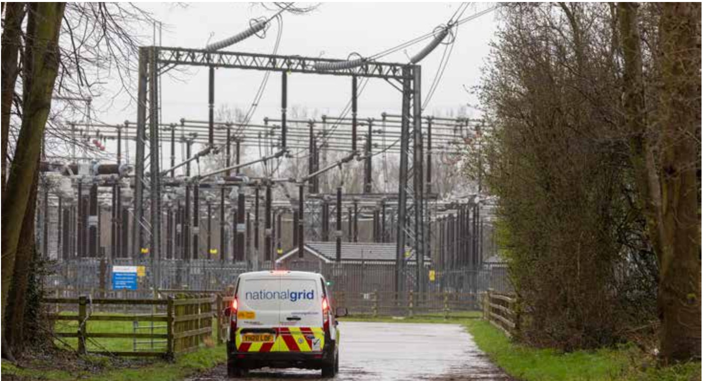
Example of a 400 kV substation for illustrative purposes only.
