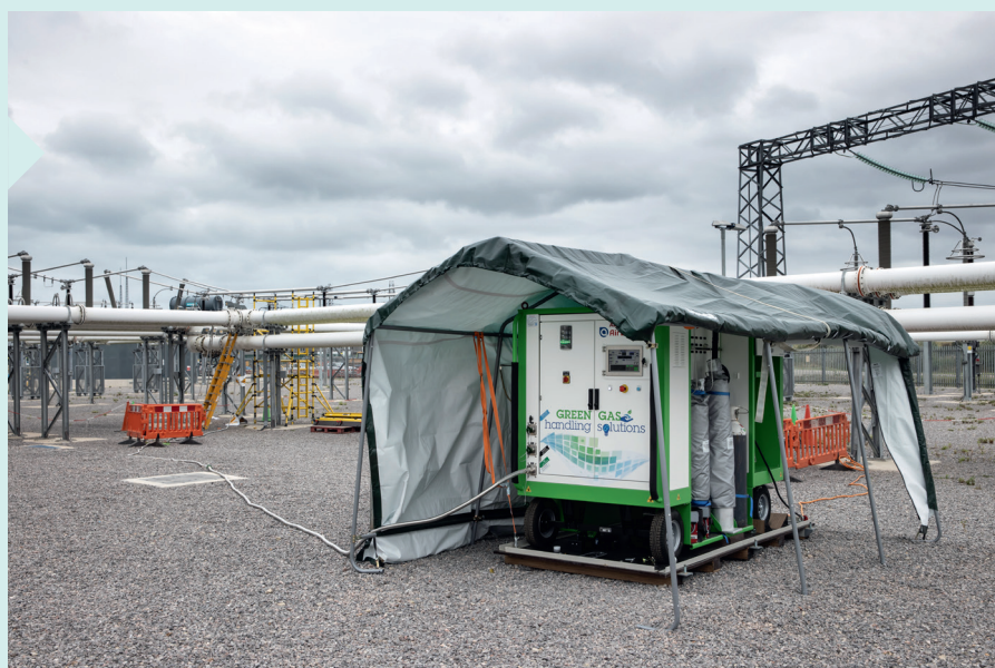
Onsite gas cart used to retro fill existing gas-insulated, high-voltage switchgear, with an alternative low global warming g 3 gas, designed for high-voltage transmission equipment, Richborough Substation, Kent, UK
