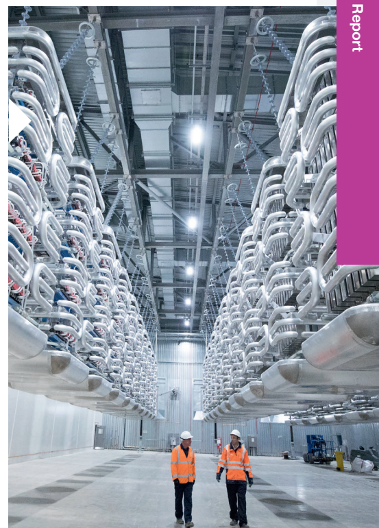
Inside the UK valve hall at NGV's 1GW IFA2 interconnector
