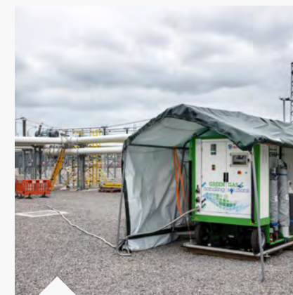
Onsite gas cart used to retrofill existing Gas Insulated Busbar with an alternative low global warming g3 gas designed for high-voltage transmission equipment
