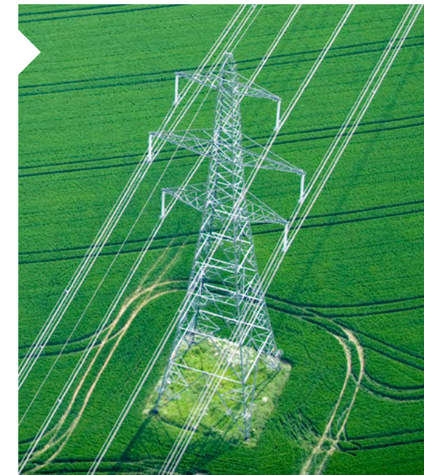
400kv lattice pylon, UK
