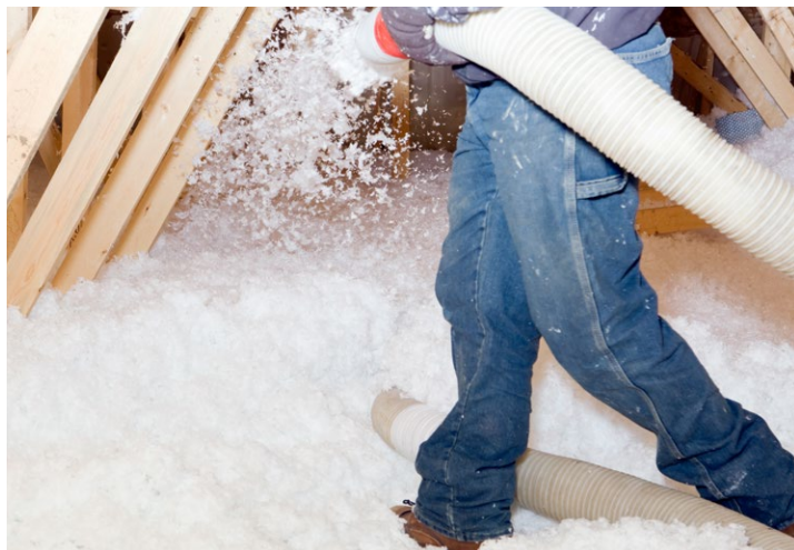
Scaling up insulation (pictured) and other buildings energy efficiency improvements are foundational to keeping energy affordable and achieving our net zero future.
