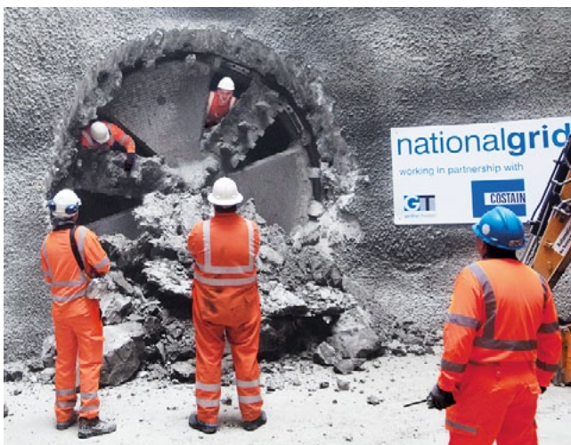
London power tunnels
