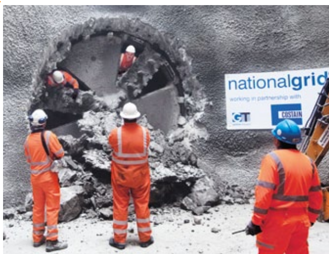
London power tunnels
