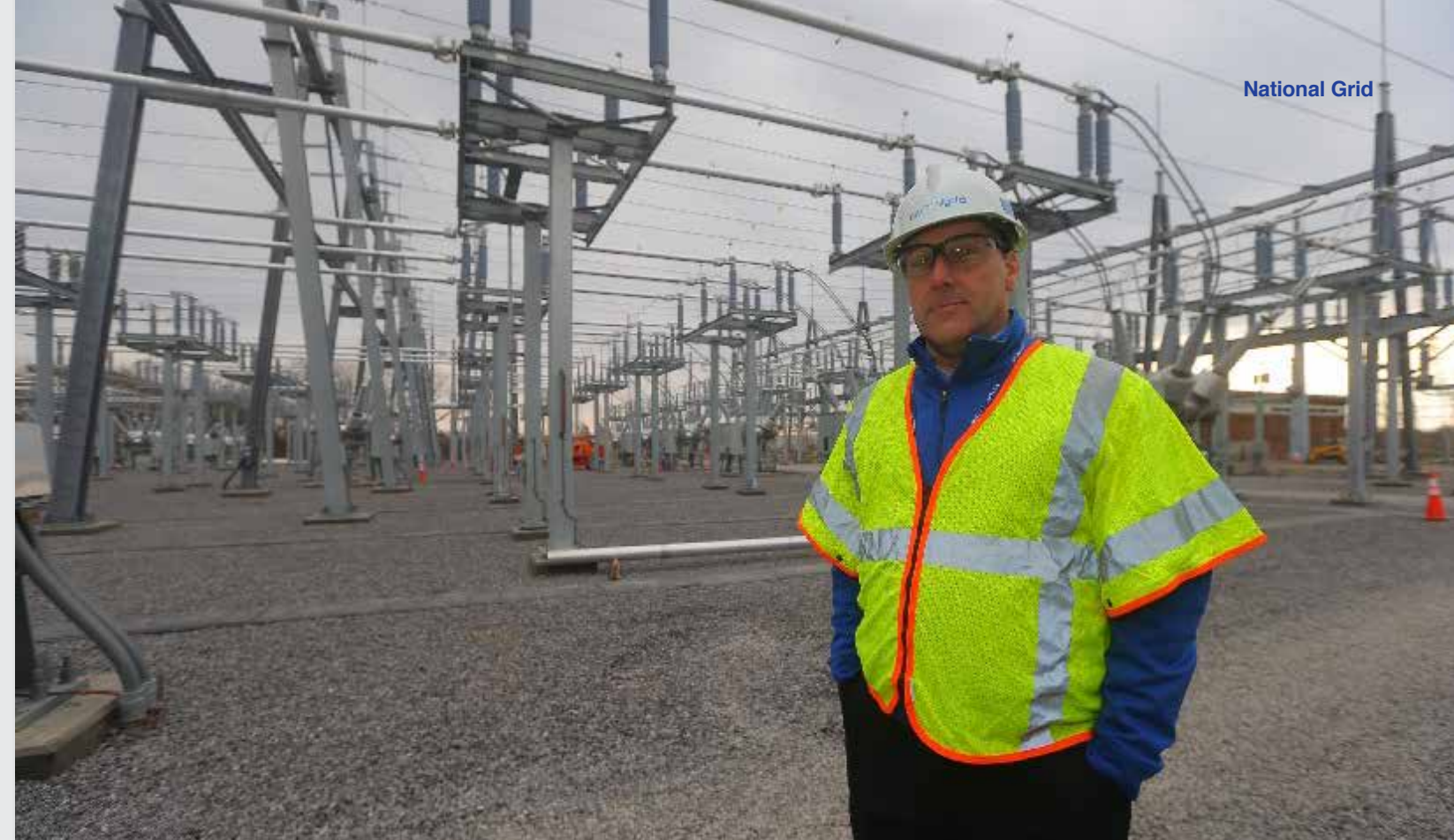
Ken Kujawa, manager, Community & Customer, at the Gardenville Substation
