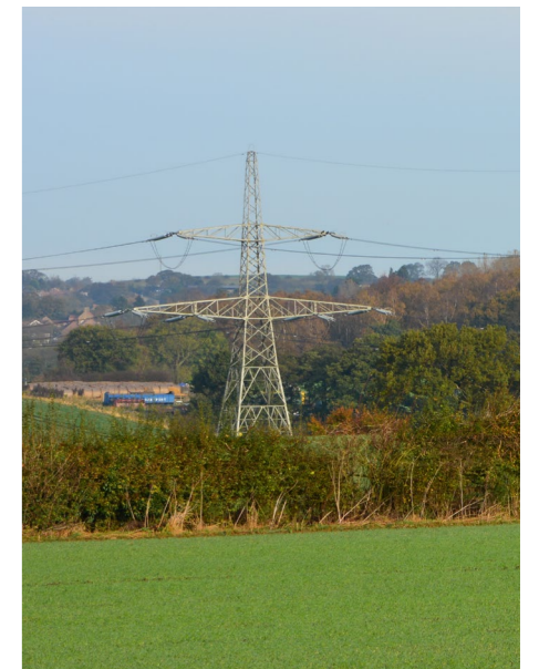
Lower height lattice pylon
