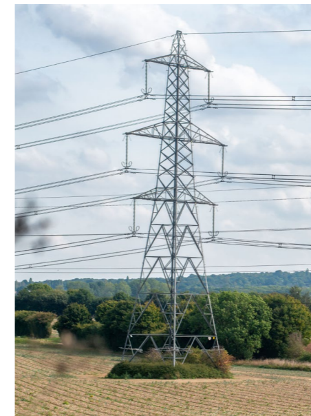
Standard lattice pylon
