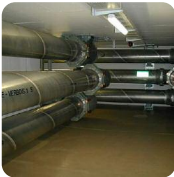
GIL installed in tunnel.
