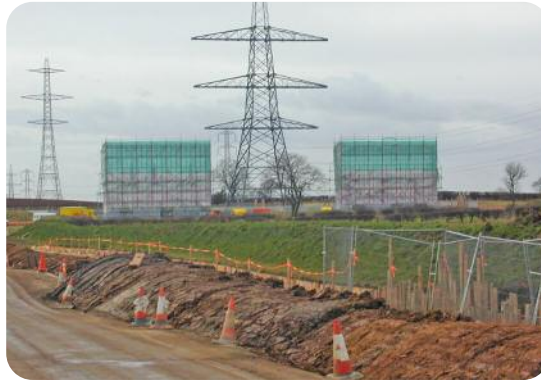
Left: A typical sealing end compound for a directly buried cable.
