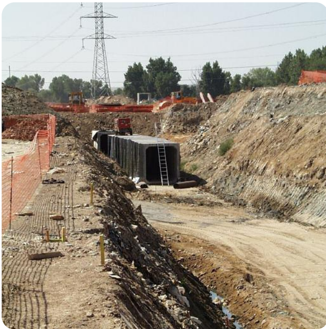
Cut and cover tunnel installation in mainland Europe. This technology is not used by National Grid.
