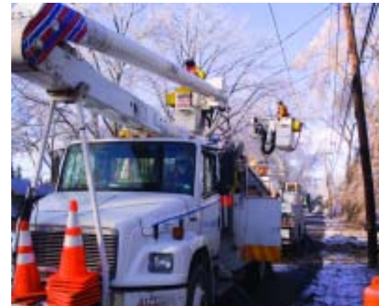
Despite cold weather and gusting winds, National Grid employees were focused on restoration efforts.
