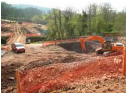
Before Construction of one of two new gas pipelines through the south west.
